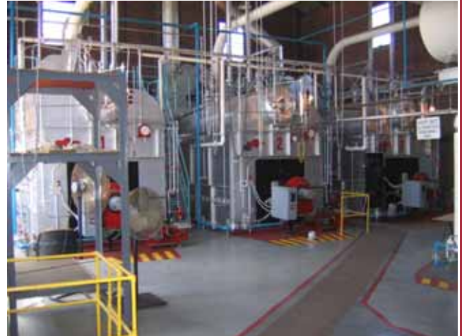
The boiler rooms at St. John's College have been the site of numerous repairs in recent years.
